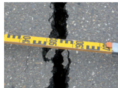
Scheur in asfalt
